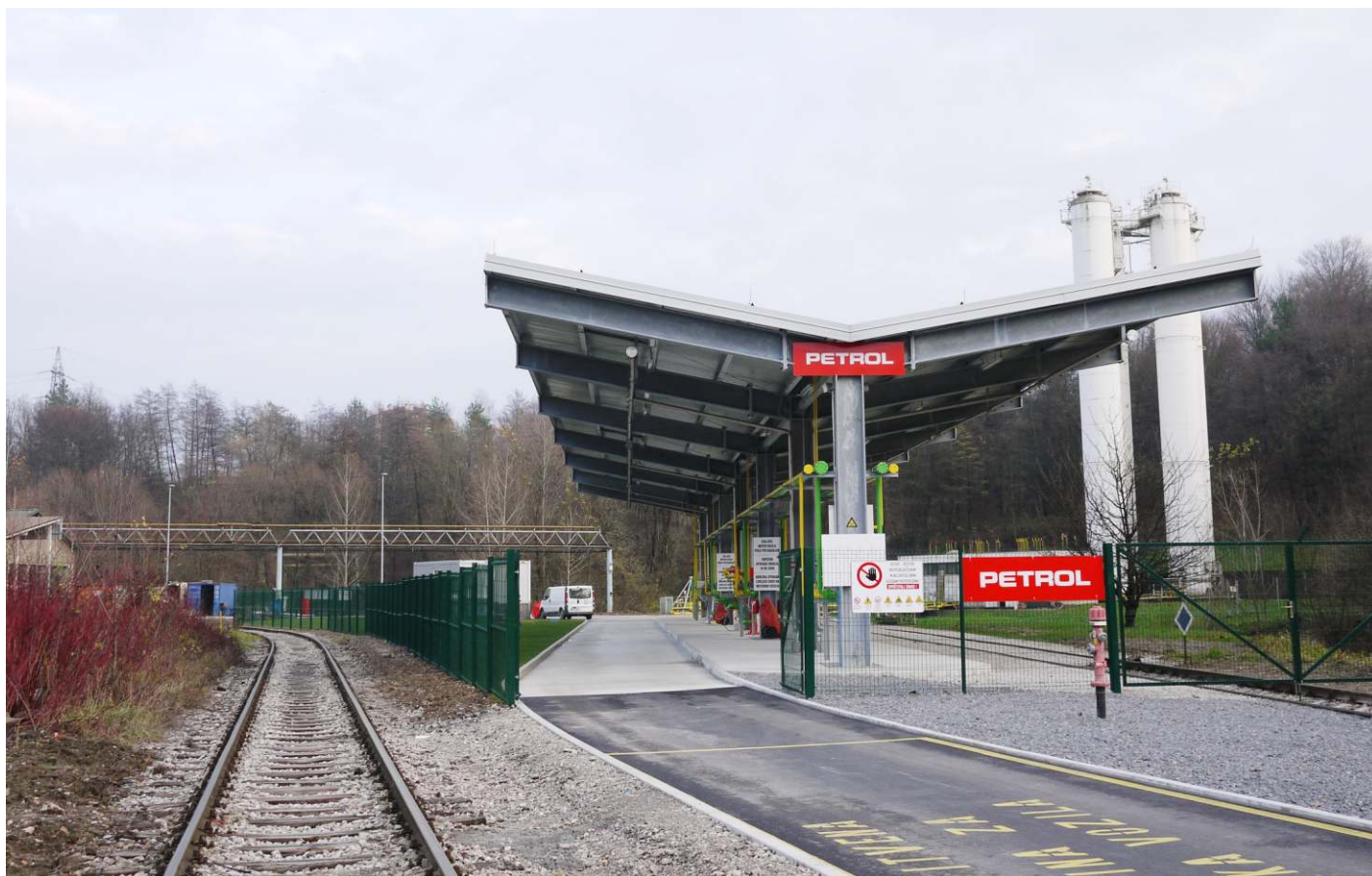
Picture above: the liquid petroleum gas decanting station;
